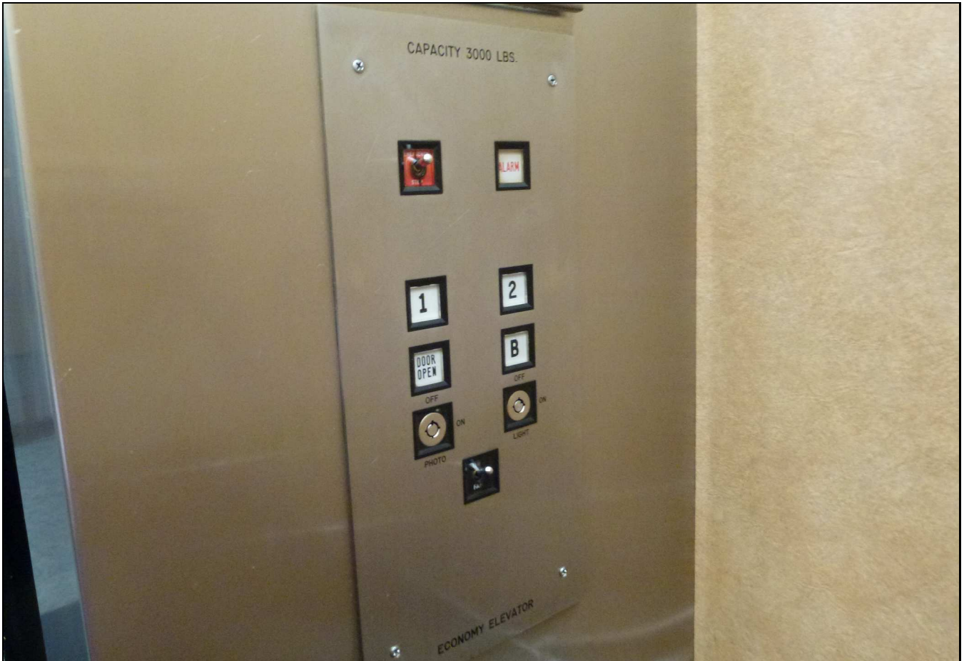
12. Elkhart Courts Bldg Elevator Buttons 2
