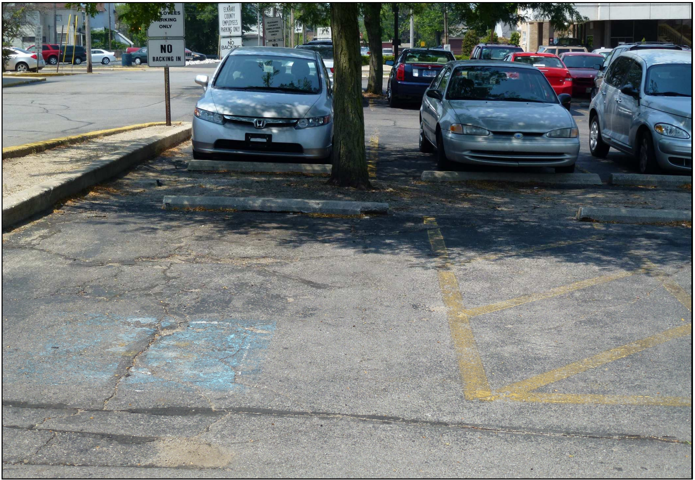
01. Elkhart Courts Bldg Handicapped Parking
